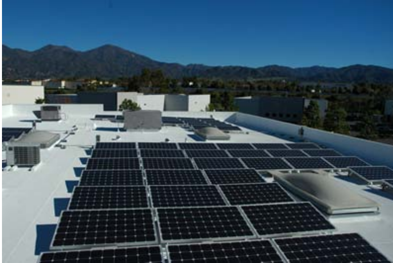
Installation of solar photovoltaic panels on a cool roof in Rancho Santa Margarita, California. Photo courtesy of Coat 'N' Cool.
